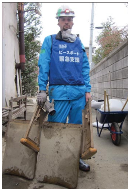
John cleaning up a cinema that had been ravaged by the floodwaters of the tsunami. He is in the protective gear required during cleanup shifts.
